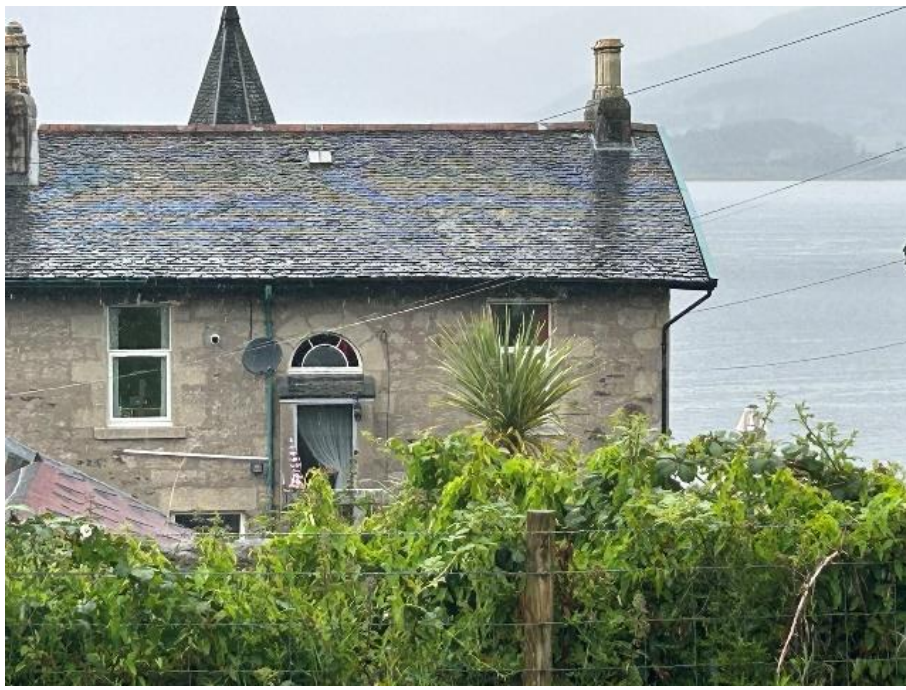
Rear elevation of 32 Crichton Road demonstrating a mixture of uPVC and timber windows
