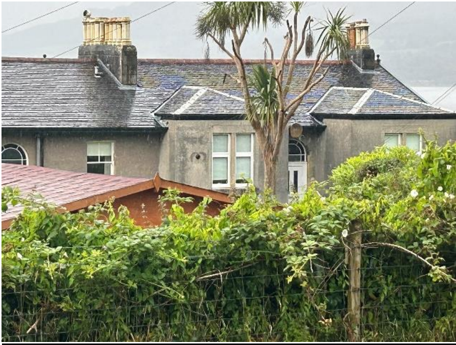
Rear elevation of 32 Crichton Road demonstrating a mixture of uPVC and timber windows.
